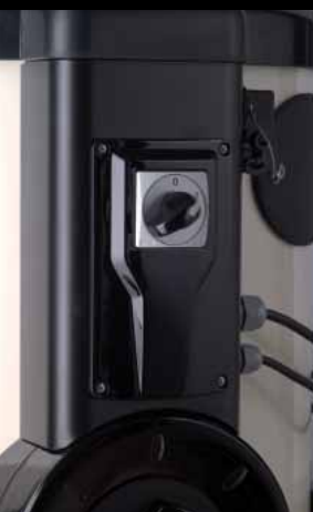
Control switch and wiring panel
